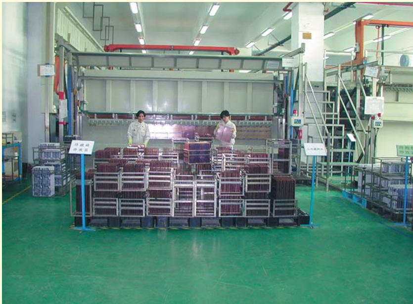
Plating tanks as big as your living room in the newly installed High Capacity Plating plant!
